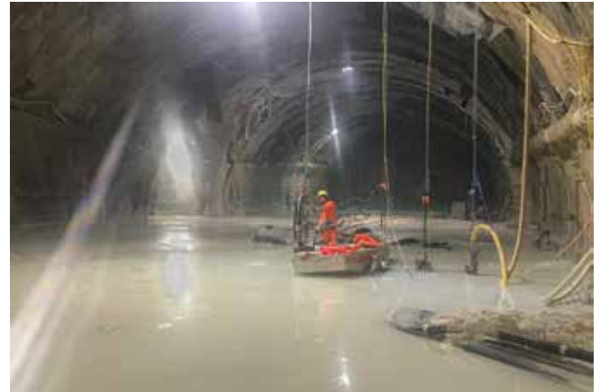
Fig. 6: Flood in the tunnel tube due to a massive water ingress.
