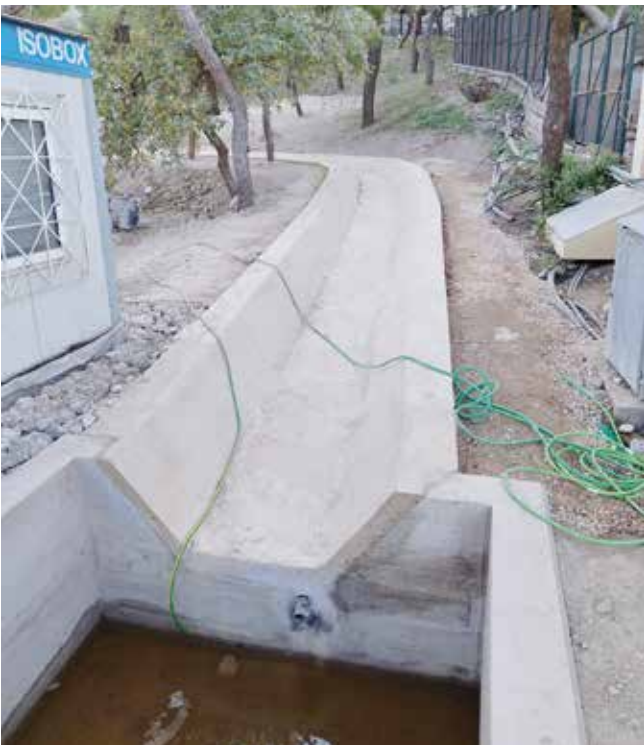
Fig. 21: A stretch of the drainage system to the north of the foot of the west end of the Acropolis. A massive channel, made of reinforced concrete for leading the water into the drain pit, seen at the bottom of the picture (2022). Photo: Tasos Tanoula
