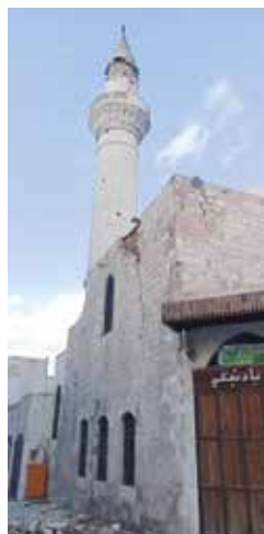
Fig. 37: Ottoman mosque: collapse of newly restored parts.
