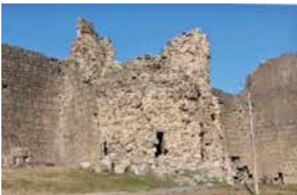
Fig. 59: 58th Tower: There are numerous falls on the surface and inside the tower walls. There are also cracks descending from the crenel window. It bears risks.
