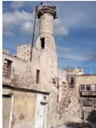
Fig. 11, 12: Great damage in a mosque in the "Aqaba" neighbourhood.
