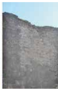
Fig. 35–37: Wall between 18th and 17th Tower: There are earthquake-induced surface collapses on the buttress and the subsequent fortification wall.
