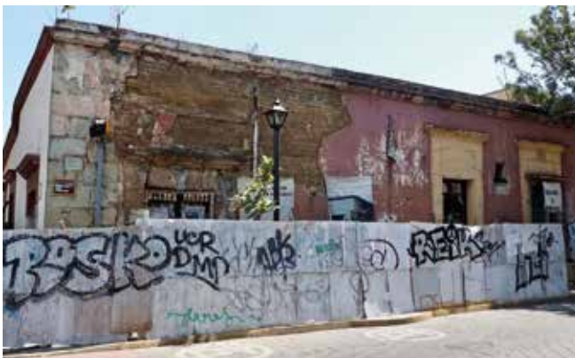
Fig. 2: Buildings' deterioration and vandalism in the historical centre.
