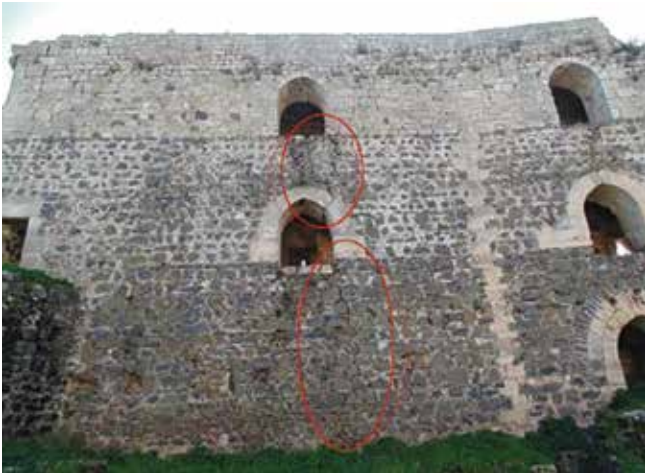
Fig. 1: Collapse of a part of the wall filling, with a height of 5m and width of 1.5m. The filling consists of limestone and basalt and traditional binding components.
