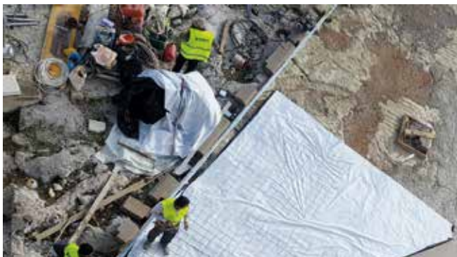
Fig. 1: The area in front of the east front of the Propylaea, in the process of being paved with reinforced concrete, covering over the face of the living rock. View from the top of the east front of the Propylaea. The metal mesh is spread on the plastic sheet spread out on the living rock.
