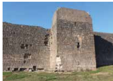
Fig. 60: 57th Tower: Stones fell down from the surface of the southern façade, and there are swellings around the fallen area. In the lower part of the southeast corner of the tower, there is previous destruction.
