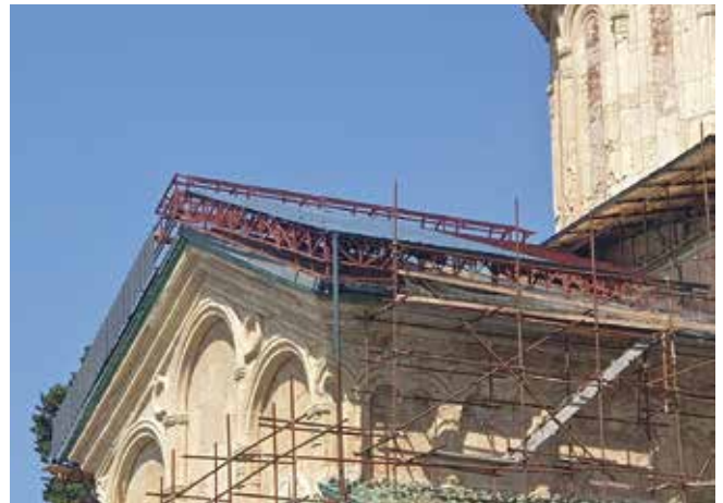
Fig. 2: New temporary roof cover on the Western arm under construction, September 2022. Photo: Europe Our House
