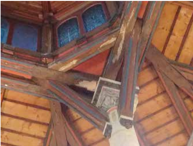
Fig. 7: Damage to the roof truss. Photo: Henning Frase
