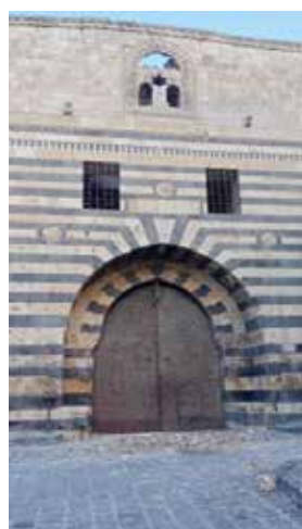
Fig. 38: Khan al-Wazir: Bulging at the top of the façade and some of its parts falling off
