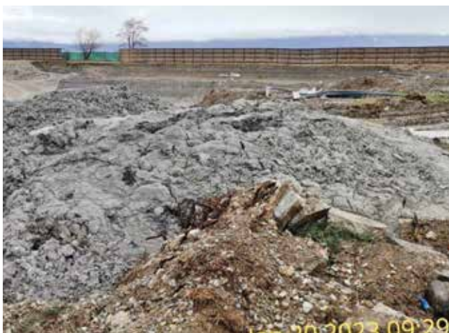
Fig. 7: A State Environment Inspectorate photo in January 2023 shows the construction site for the new, legally-disputed hotel that is being built at the former Restaurant Park. It will encroach on Lake Ohrid's 50m Green Belt Zone.
