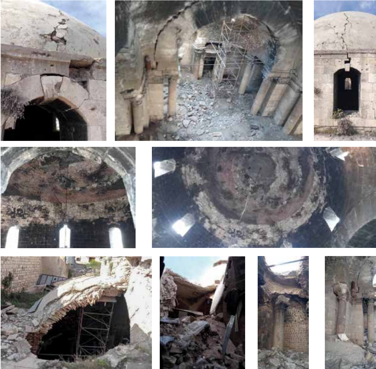
Fig. 27–35: Significant and dangerous damages in "St. Helena's Church".
