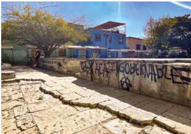
Fig. 5: Damages to Plazuela del Carmen Alto.
