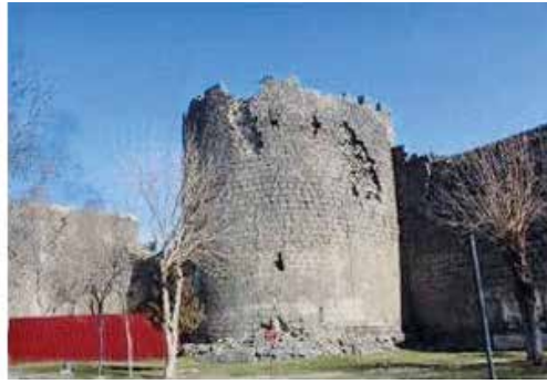
Fig. 19: 23th Tower: There are swellings and jointing discharges at the areas where the surface stones were previously destroyed. It possesses risks. In addition, there is a risk of stone spills due to jointing discharge in dendan residues.
