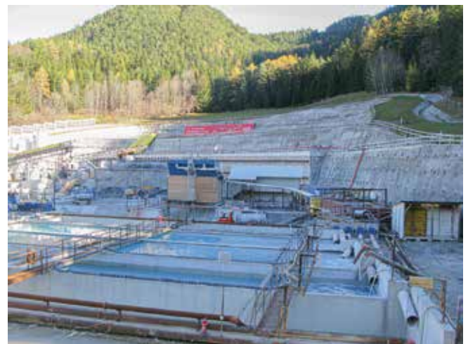
Fig. 7: At the Göstritz SBTn intermediate intervention near the Maria Schutz pilgrimage site, groundwater drained from the mountain massif is collected in settling basins. According to media reports, this currently amounts to around 10 million liters of water per day. After completion of the Semmering Base Tunnel, 38 million liters of water are to be drained daily in the long term and removed from the natural water balance of the Semmering. It is feared that the Semmering region will sooner or later be karstified.
