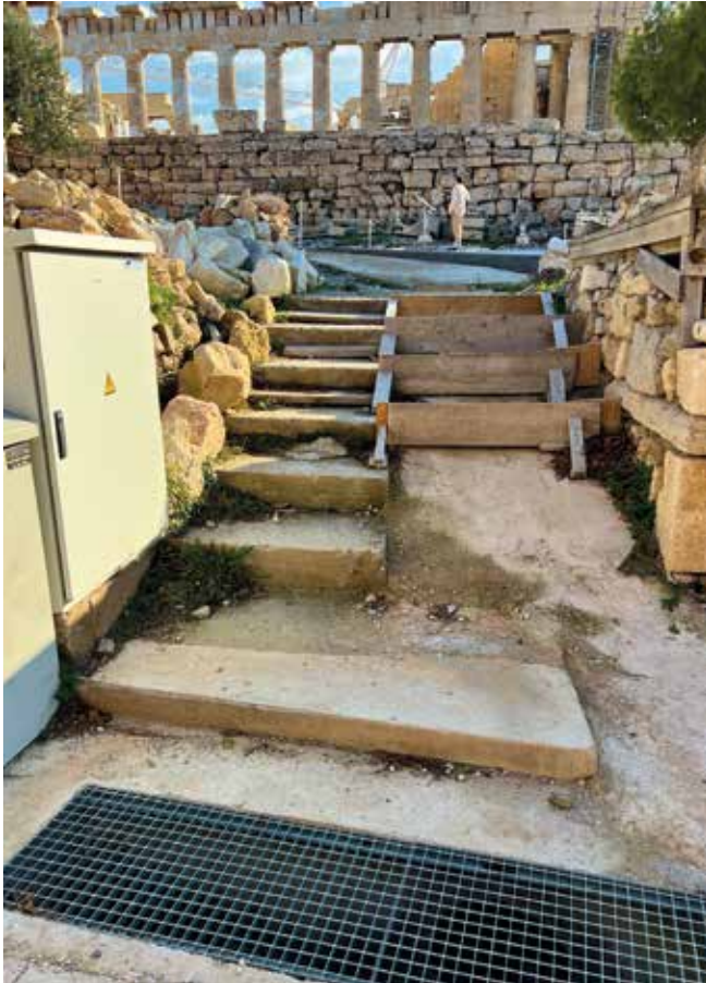
Fig. 14: Same view as in Fig. 13, in January 2023. The pipes are covered with the concrete ramp bearing wooden planks, the formwork for shaping concrete steps to lead from the upper level (which in Fig. 12 is being paved with reinforced concrete), to the lower level illustrated in Fig. 15, 17.
