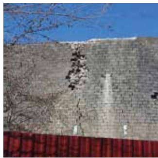
Fig. 20 and 21: 22nd Gate - Urfa Gate South Tower: On its southern façade, there is a crack that runs from top to bottom. The crack's decomposition continues beneath the surface and on the infill wall. There are also swellings on the surface of the tower. Several new
