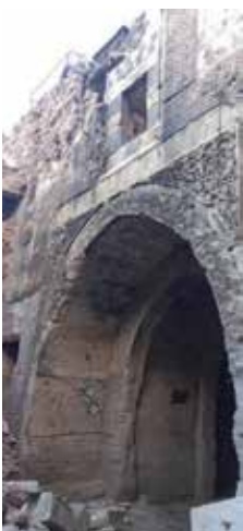
Fig. 36: Khan al-Sabun: the collapse of the main façade decorations
