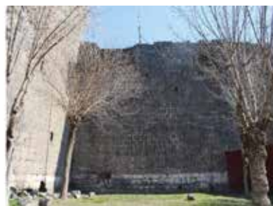
Fig. 22: Wall between 21st and 20th Towers: Several new stone falls have appeared in areas where surface stones were previously poured. The risk of stone spills persists.
