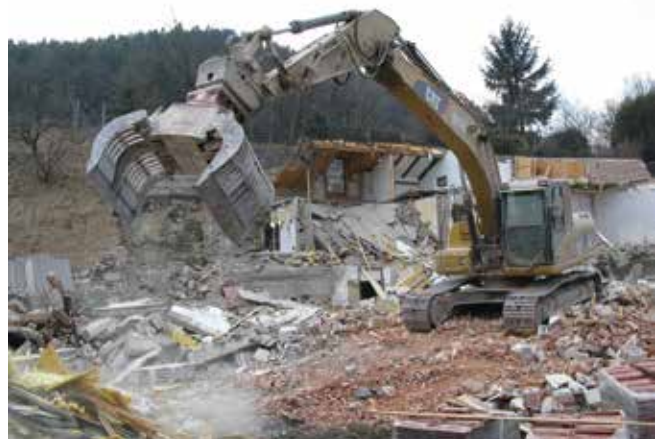
Fig. 3: For the construction site and the future north portal of the Semmering Base Tunnel, an entire district of Gloggnitz was razed.
