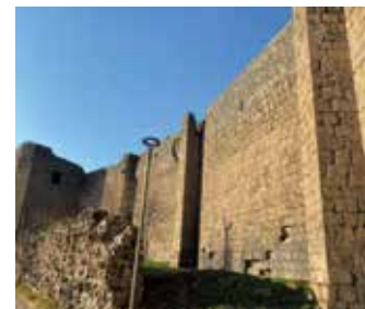
Fig. 61: Wall between 52th and 51st Towers: A decomposition occurred at the joint of the second buttress and the wall. Moreover, there are cracks on the buttress. It is at risk.
