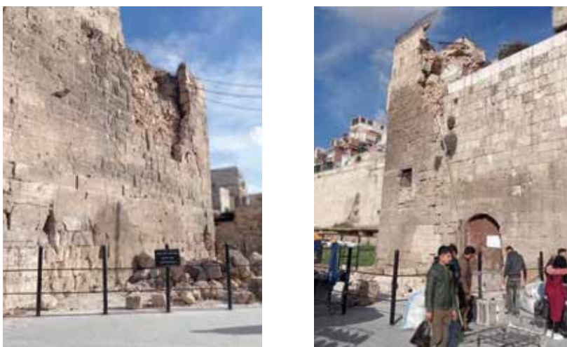
Fig. 8, 9: Collapses and cracks in parts of the "Antioch Gate".
