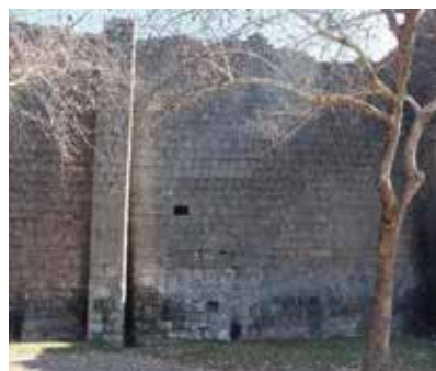
Fig. 15, 16: Wall between 25th and 24th Towers, 10.02.2023: A stone fell from the secondary wall gate, located on the wall, which was closed, and there is a joint opening of the buttress from top to bottom. Stones may fall from the observation unit ( dendan ) ruins. Risky.
