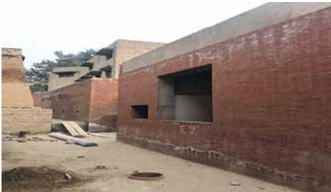
Fig. 2: The new fine dining restaurant under construction, only a few feet away from the historical Royal Kitchen (left), 2018.
