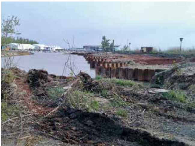
Fig. 1: Steel structures placed during the construction of villas in Neusiedl am See. Photo: Rudolf Golubich
