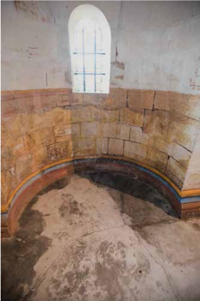
Fig. 6: Moisture and cracks in the floor of St. Ulrich's Chapel. Photo: Henning Frase
