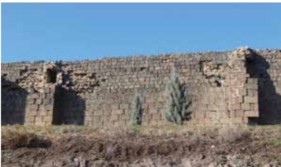
Fig. 57: Wall between 61st and 60th Towers: Slits occurred on both buttresses and bear risks.
