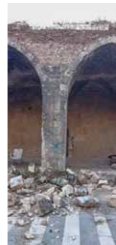
Fig. 39: Partial collapse in many cases
